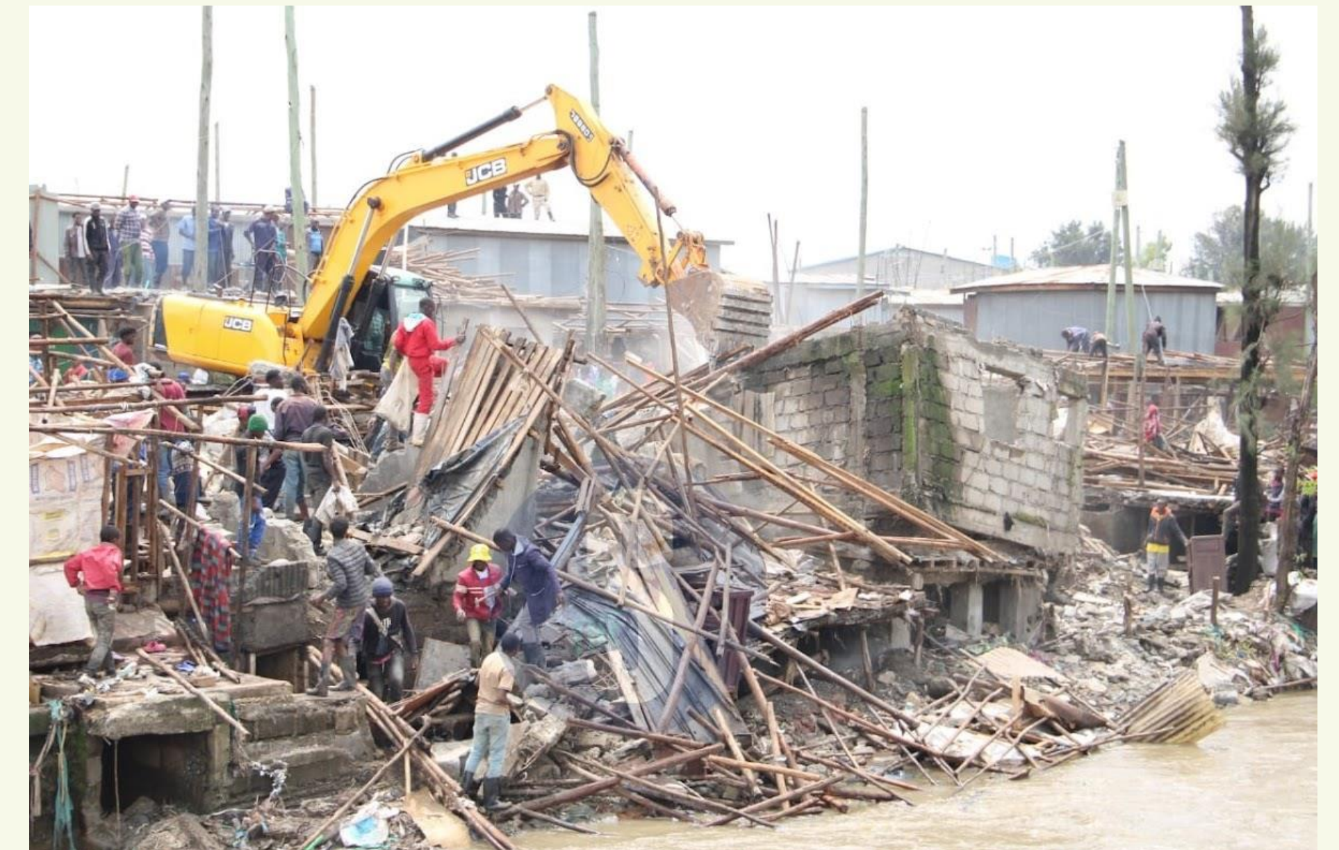
Demolition of urban poor settlements along Nairobi Rivers amid Floods in April-May 2024. Image © anfoz.com
