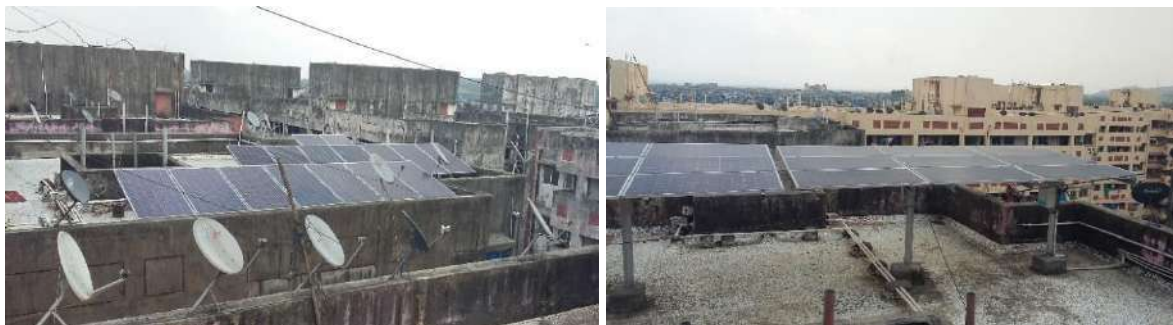
Figure 3: Solar panels installed in the rooftop of the buildings
