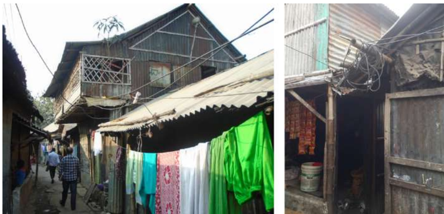
Figure 5: Unsafe electrical cabling (M Jones and S. M. Younus)
