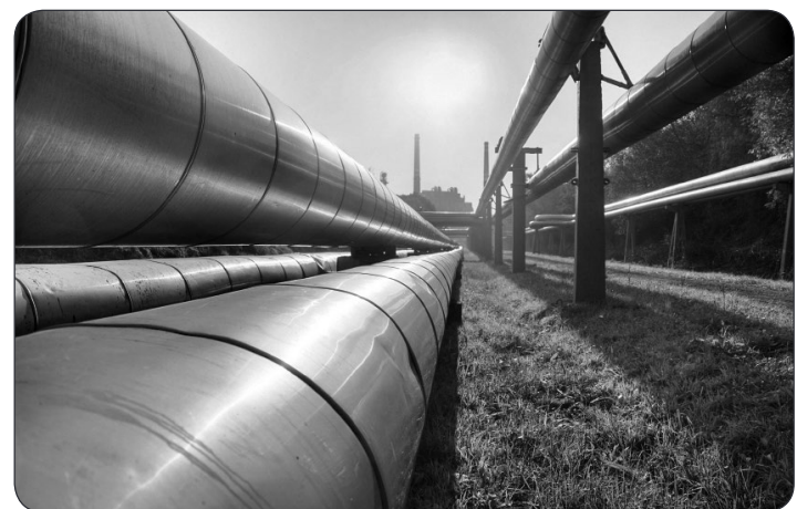
Hydrogen can be transported via pipeline, truck, rail, and barge.
